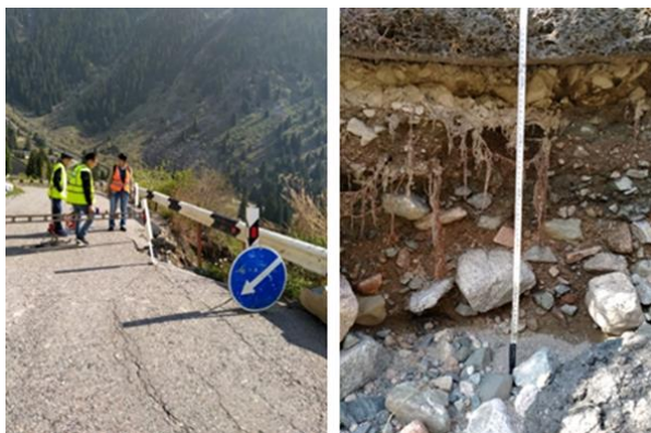
Fig. 4 – The erosion of the grading slope because of a faint provision of the road pavement's drainage
