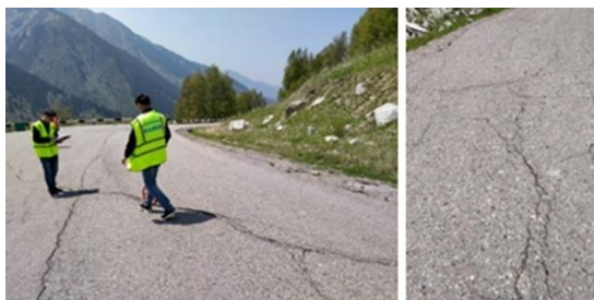
Fig.2 – The longitudinal cracks on the road pavement
