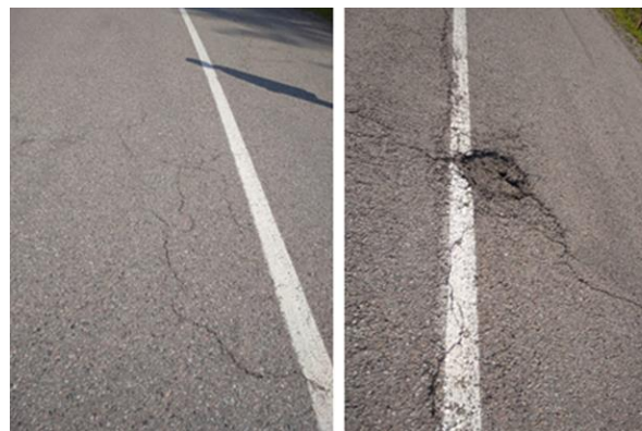
Fig. 5 –The tiny cracks and holes on the fifth testing site
