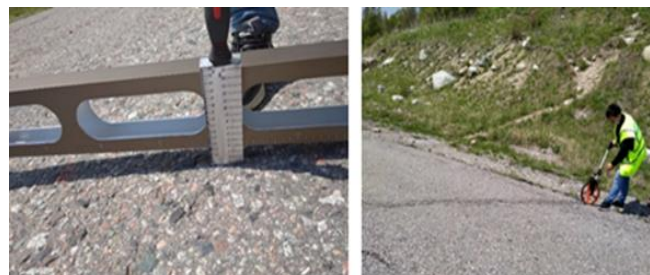
Fig. 3 – The road unevenness and deep transversal cracks
